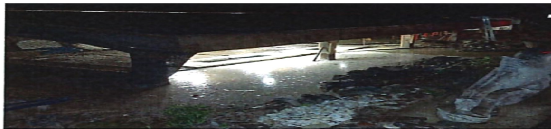
DCH captrough area flooded
