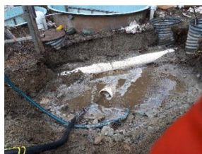
Broken pipe at DCH facility April 2019
