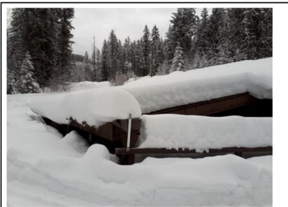
Snow load on top of DCH building
